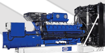
FG WILSON GENERATOR
